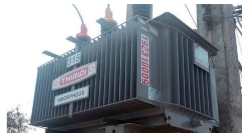
Introduction of Amorphous High Efficiency Transformers in Power Grid, Yuko Keiso Co., Ltd., ①Vietnam, ②Lao PDR
