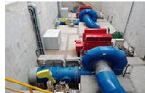
Hydro Power Plant, Toyo Energy Farm Co., Ltd., Indonesia
