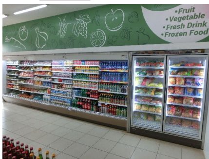
Energy saving at convenience stores, Panasonic, Indonesia
